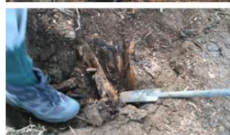
Jack hammer needed to remove buried root at Gate 231
