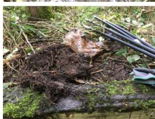
The roots, plastic bags and weeds that were causing the blockage and flooding.
