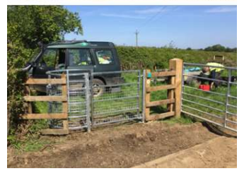
Reverse views of Gate 167 before & after. Note normally locked seven bar steel field gate.
